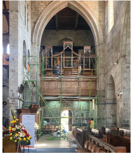
Empty casework, awaiting return of the pipes (photos provided by Michael Farley)
